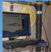
Computerized energy management control system provides 24-hour monitoring of all mechanical and plumbing systems.
