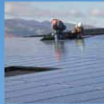
97 KW grid-connected photovoltaic solar power system
