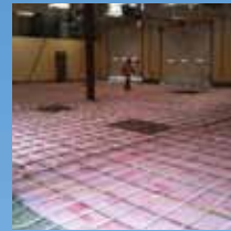
Radiant floor heating system in maintenance building
